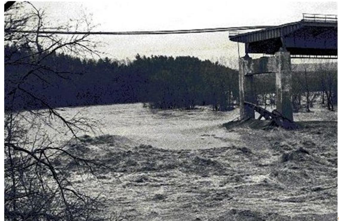
The collapse of the I-90 Schoharie Creek Bridge, New York due to scour
