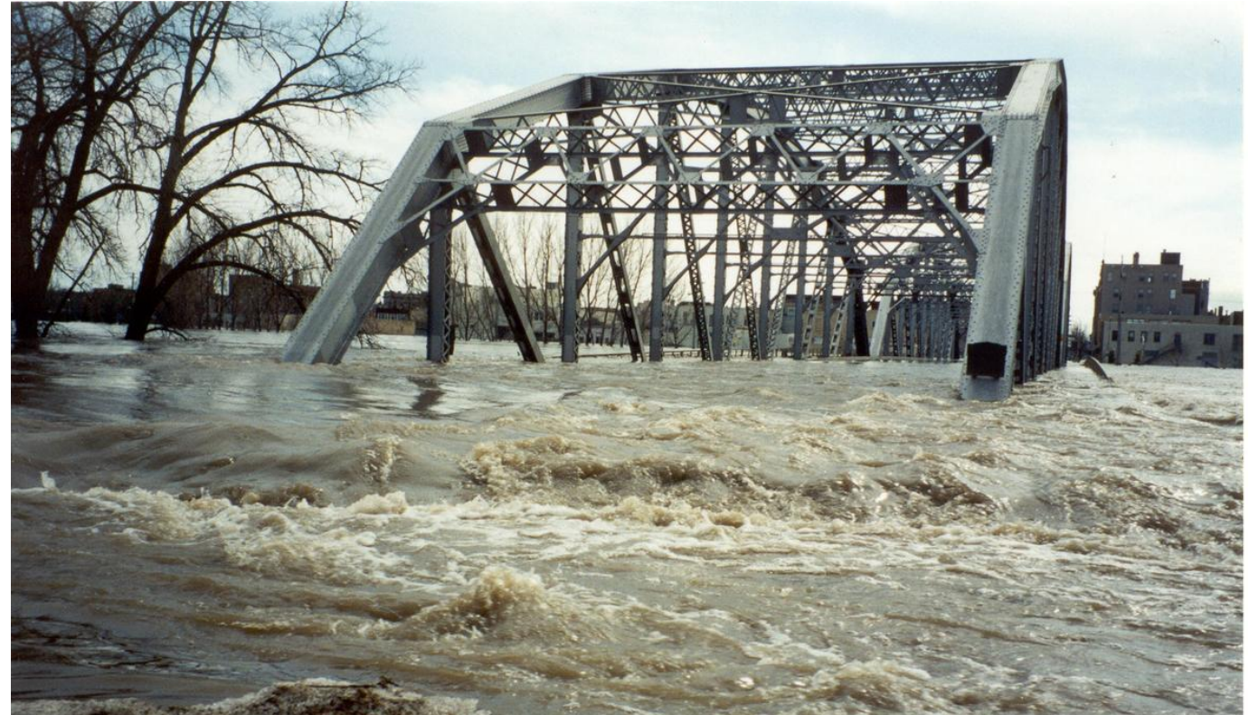
Flooding of a bridge during the 1997 Red River of the North flood, Minnesota, U.S.A.
