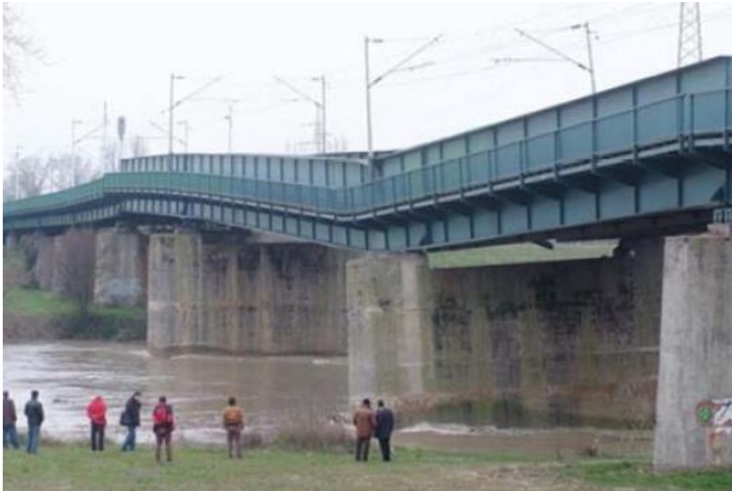
Failure of Sava bridge, Zagreb due to scour
