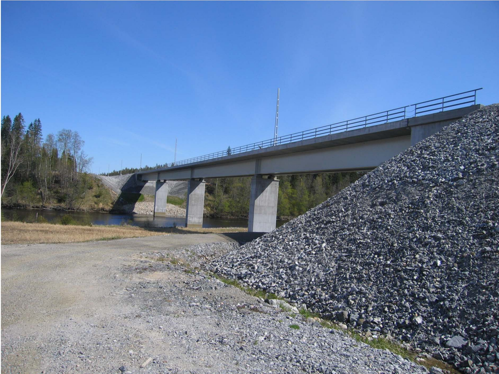
A steel girder railway bridge. To the right, the erosion protection of the slope is shown.
